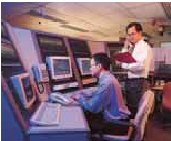
The Computer Room which houses the central computer system.
