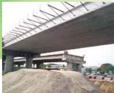
Excavation works for the 2nd phase of the PJS 8 underpass at Bandar Sunway.
