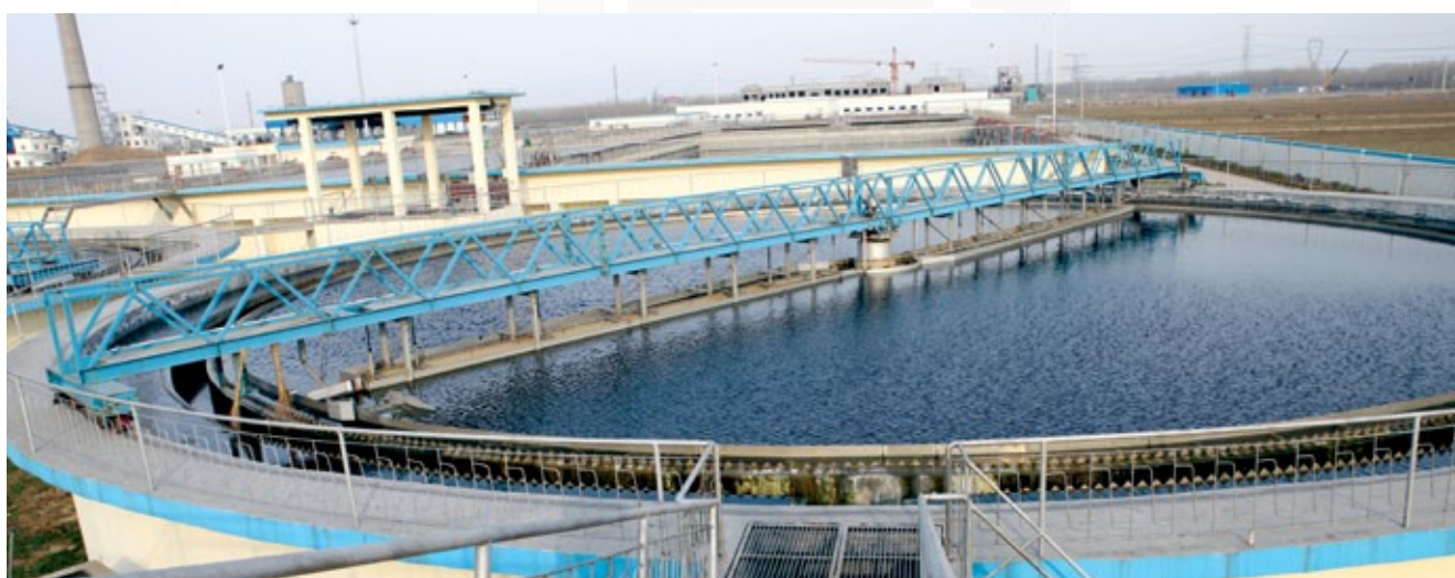
Secondary sedimentation tank of the DSG Taian Sewage Treatment Plant in the People's Republic of China.
