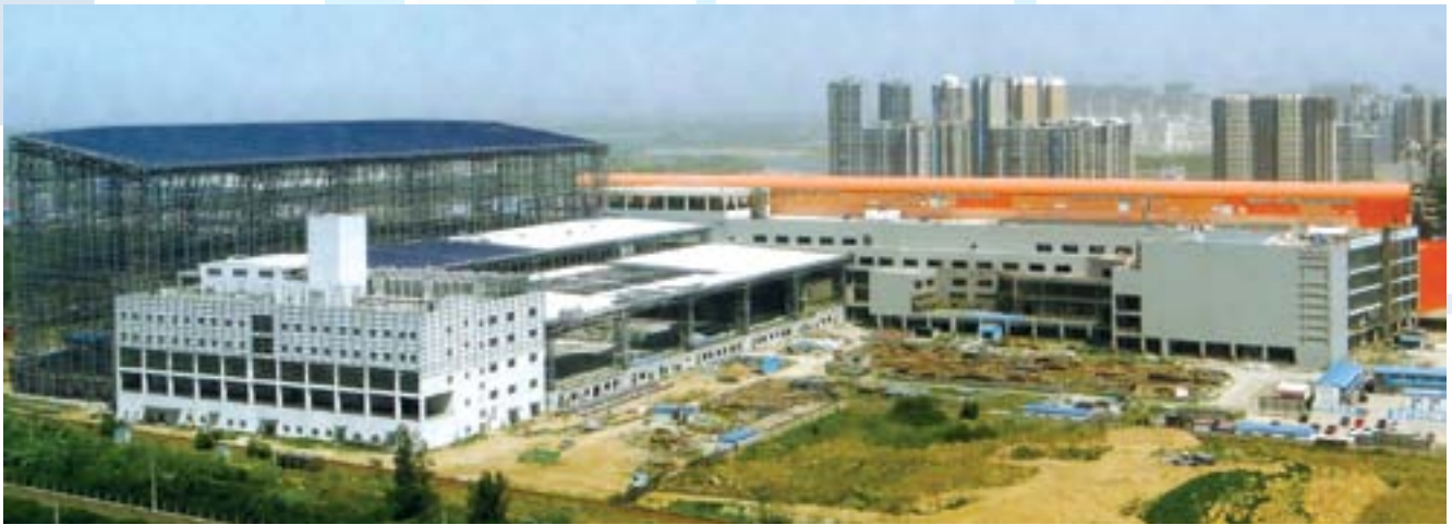
Great Mall of China, Beijing, People's Republic of China - construction in progress.
