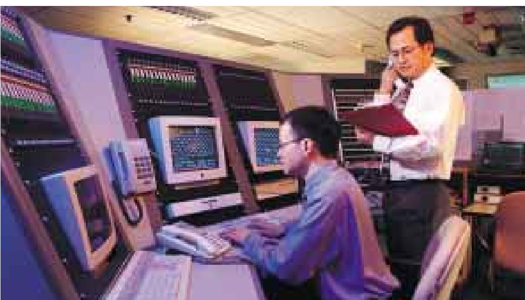
Communication Control Console, which controls the entire data communication network.
