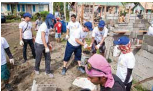
Paul Soo (center) carrying a pail of mixed cement to other workers.
