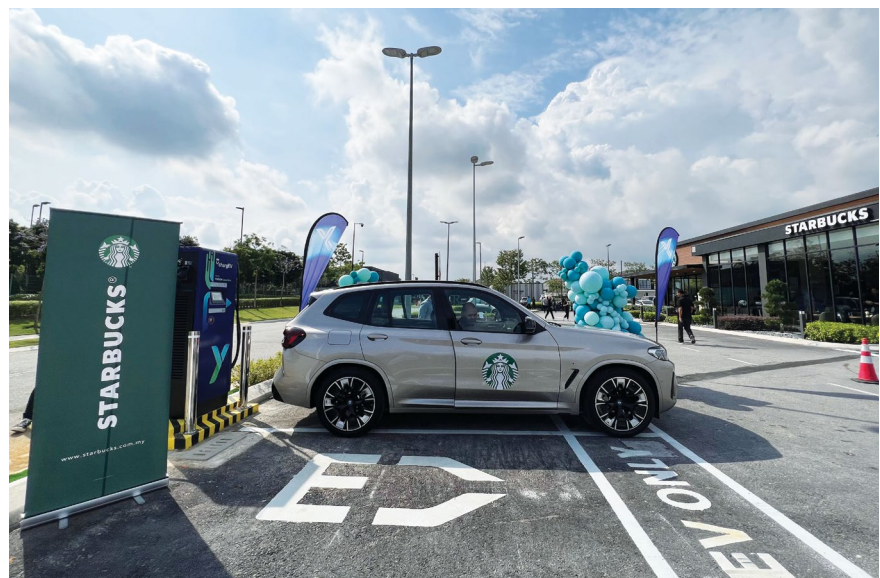
EV charging equipment in BStarbucks Drive-Thru stores.
