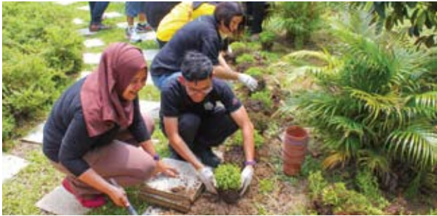
BStarbucks' partners (employees) with volunteers from Roots & Shoots Malaysia worked together to build a drainage system and landscaping project for the Community Computer Centre in Kampung Lubuk Jaya.
